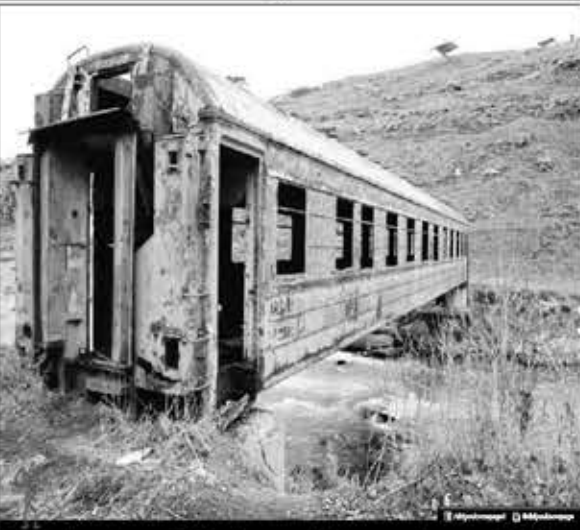
An abandoned Train coach is used as a Bridge. This is the Best Example of Recycle. Instead of Wasting Money and Sources, we should focus on things which can be reused!
